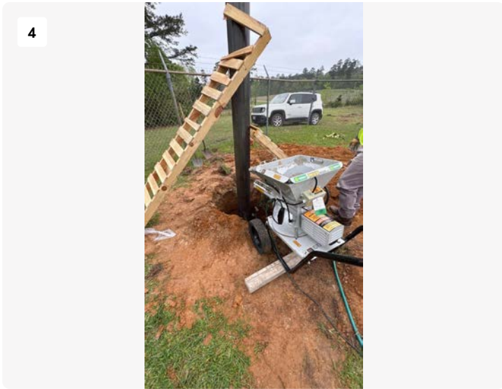
8" Schedule 40 pipe in concrete
